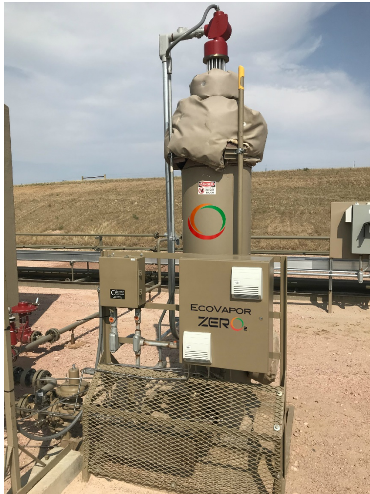
Figure 5: Oxygen Removal Unit on a Production Site
